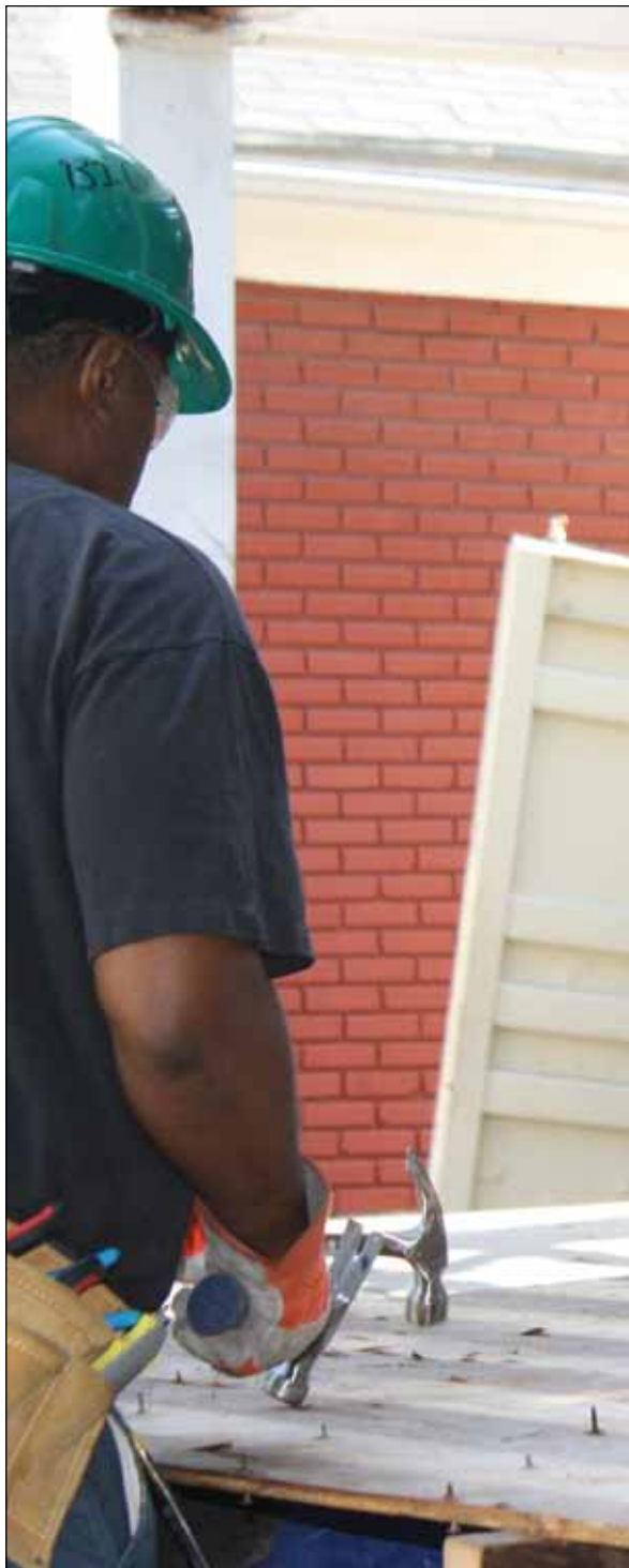
Fifteen residents received hands-on training in deconstruction of a home at 4429 Garfield, along with two days of OSHA-10 classroom training. Before the project was complete, one of the 15 had secured a union job.
